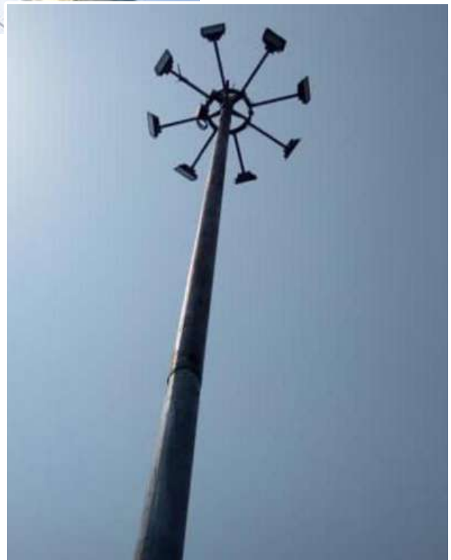
Installation at Ultratech, Hirmi, Raipur (C.G.)
